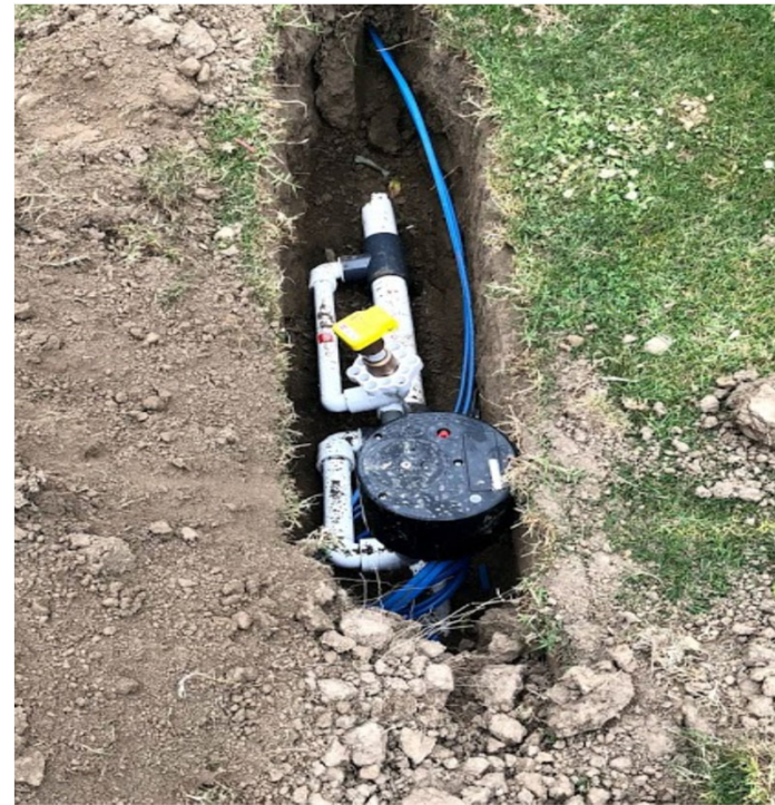
Efficient New Sprinklers
